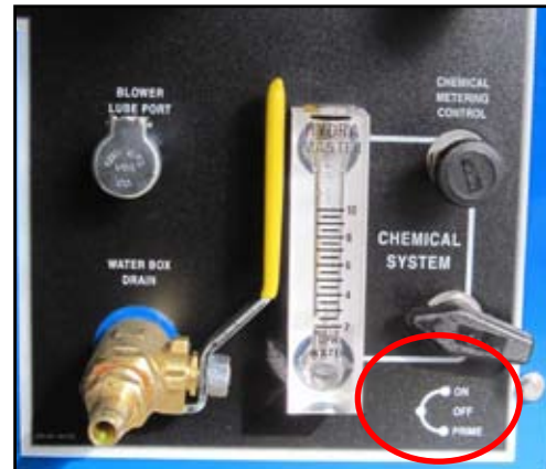
Figure 4-6. Location of Chemical System Switches
