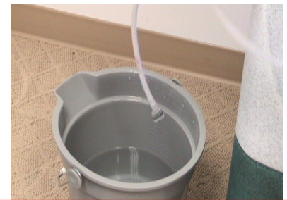
Place Chemical Feed Hose into Rinse Solution
