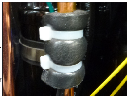
Figure 6: Thermistor attached to the refrigerant line.
