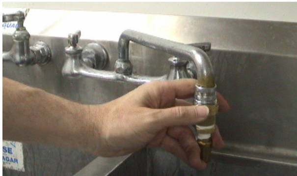
Connect the Auto-Fill Water Supply Hose to a faucet and turn on the water
